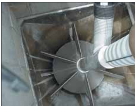
DynaSand Filter modules in concrete basin
